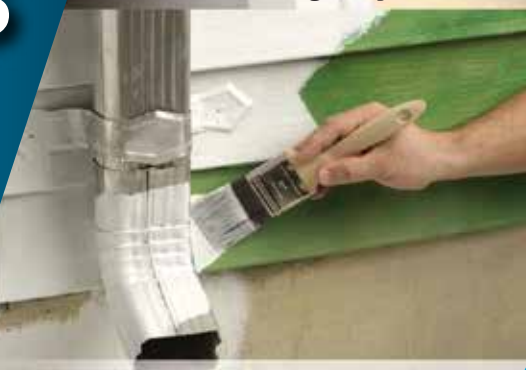
Chalky siding, masonry, metal
